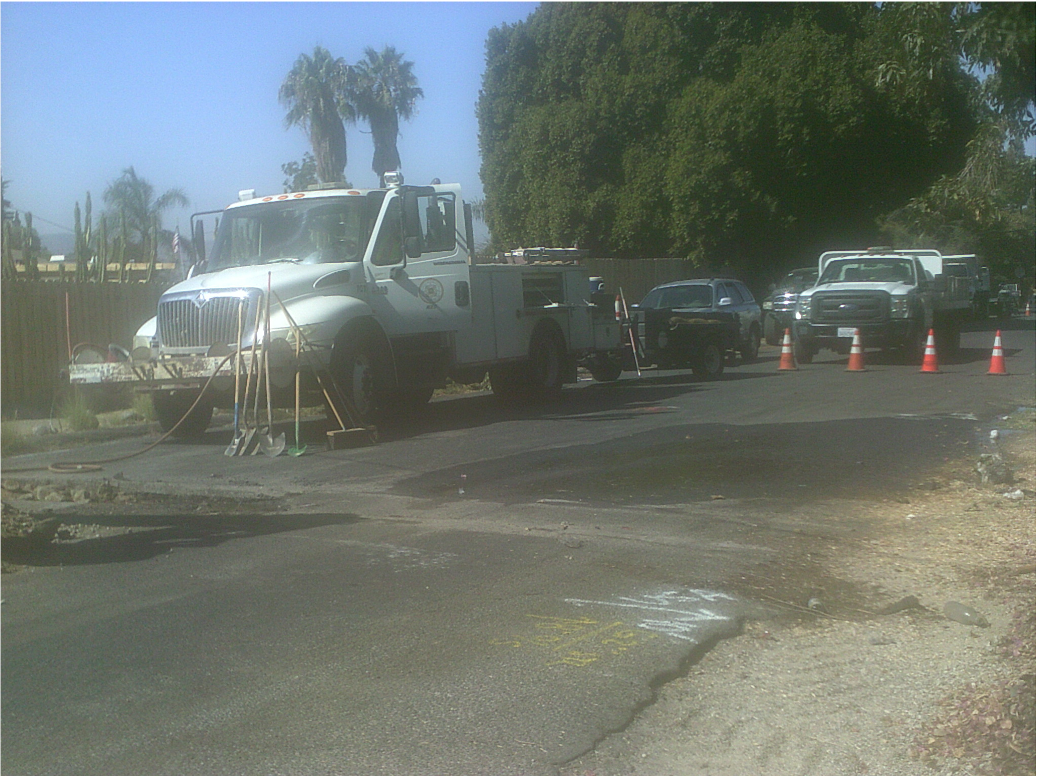
The small water “gusher” in the middle of the street.
